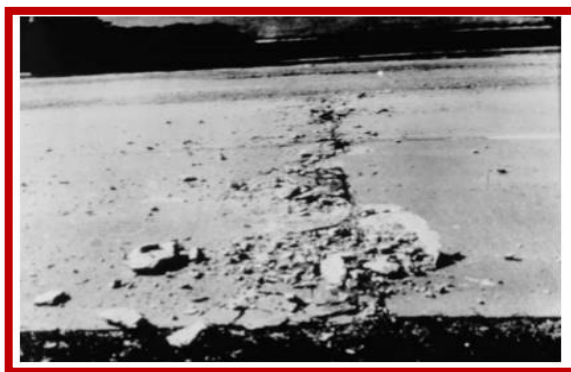
Figura 58: Blowup - Buckling - severidad media
