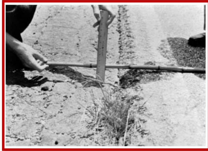
Figura 29: Desnivel carril/berma - severidad media
